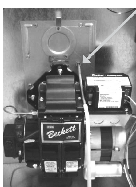
Over-fire draft access port.
