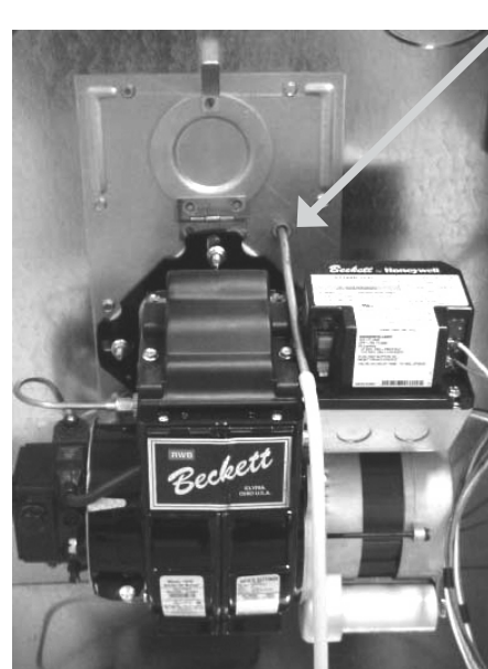
Over-fire draft access port.
