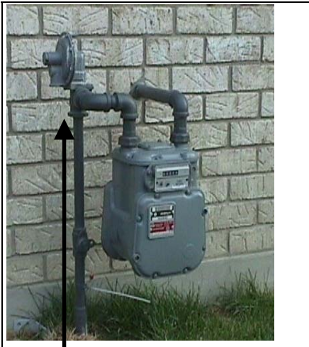
FIGURE 2: GAS REGULATOR VENT
