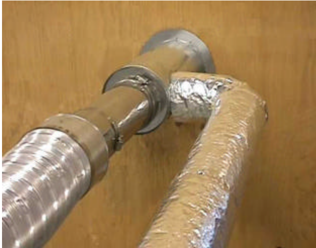
INSIDE VIEW OF VENT TERMINAL
